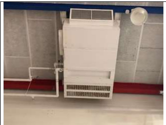
5. View of air handling unit in gym.
