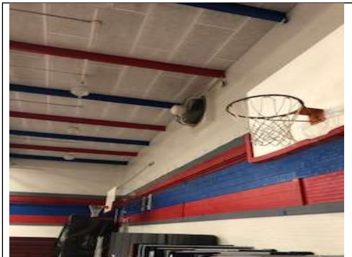
4. View of ventilation fan.
